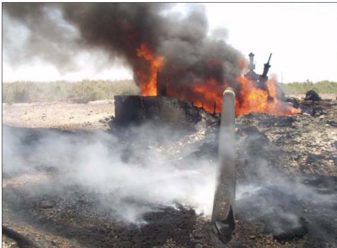
An Iraqi pipeline valve station burns prior to OPC extinguishing the blaze and beginning repairs (Fig. 3).
